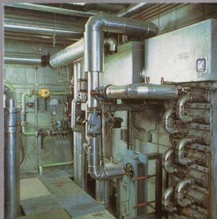
Heat exchangers for flue gas etc.
