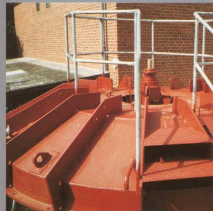
Top cover on vacuum tank
